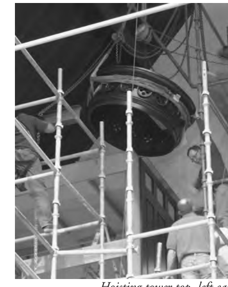
Hoisting tower top, left case
